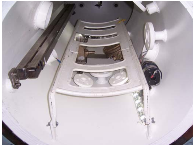
Photograph 5 - Two Six LED Lighting Systems Installed in SES Test Bed Escape Tower
